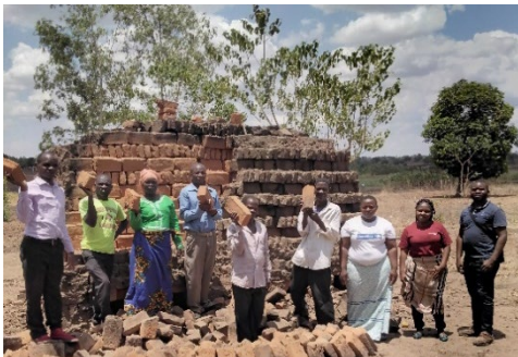
Faith leaders and SCOPE project staff displaying burnt bricks for the Mtsonthe Village Clinic construction project.
